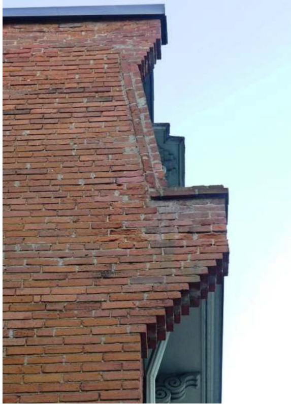
17. 193 Mutual Street : showing the corbelled firebreak wall at the second and mansard levels. ( Heritage Preservation Services, 2014 )
