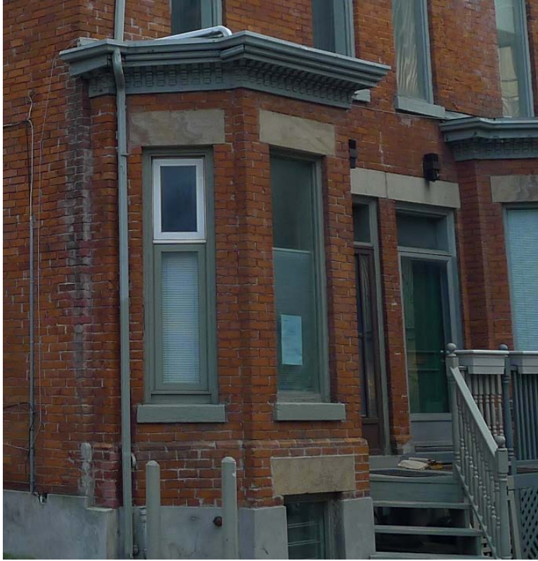
19. 193 Mutual Street : showing original surviving window pattern and proportion with the long lower sash and squarer upper sash in first floor bay window. ( Heritage Preservation Services, 2014 )
