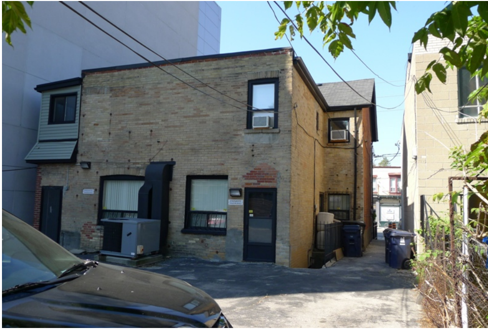
13. 811 and 813 Broadview Avenue, rear wing : showing the rear wing clad in yellow stock brick with a sloping flat roof. On the right, the side wall of the main house of 813 Broadview Avenue, clad in red brick with a gable roof. Note the later additions at ground and upper floors at 811 Broadview Avenue on the left ( Heritage Preservation Services, 2015 )
