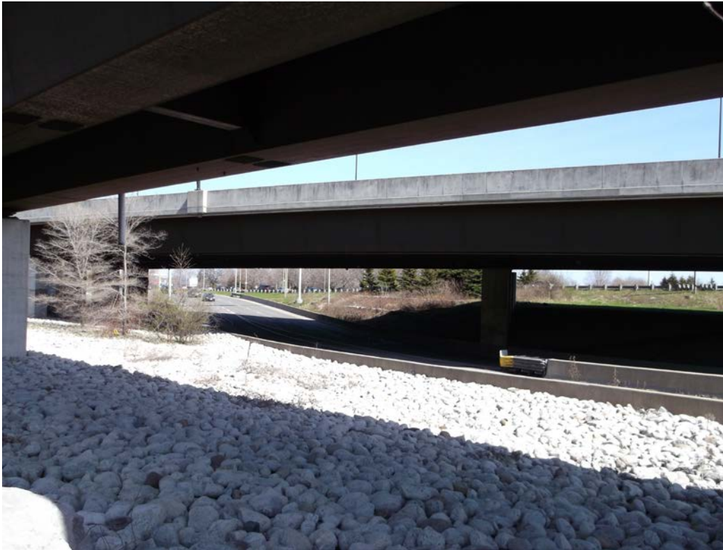
5) Humber River - East side, line-of-sight for track grade or bridge alignment, looking southeast
