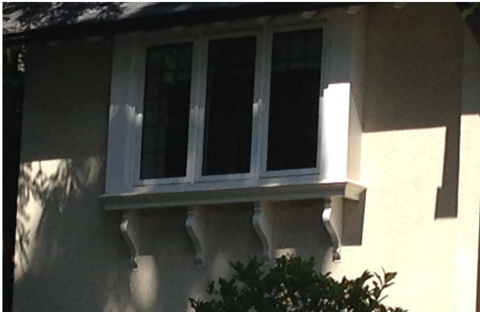
28. South elevation, oriel window detail of the west extension. The newer window maintains the details including the scroll brackets, the tripartite division and the leaded glass, but has omitted the horizontal division with upper transoms ( HPS, 2016 )
