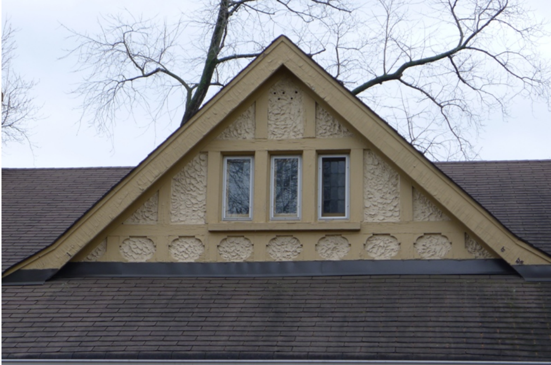
10. Page House, gable dormer, north elevation : showing the half-timbering and stucco as well as the leaded glass windows all associated with the Tudor Revival style. (HPS, 2016)
