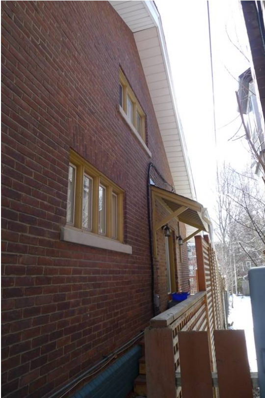
16. Page House, side (west) elevation : showing the location of the modification to the arrangement of windows in the kitchen under the hood roof. (HPS, 2016)
