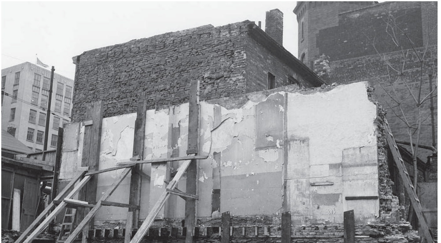
(Above) Building wall being supported during an excavation as part of the Yonge subway line construction, photo taken in 1952.
