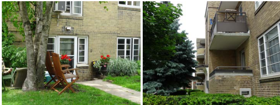
East (rear) elevation of Building A (left), and part of the west elevation of Building K on Bayview Avenue (right).
