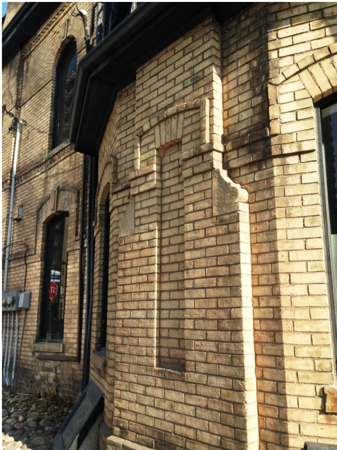
30. 79 Shuter Street, west elevation: showing the brick details, string courses, and the stone keystones, relief panels and chimney mouldings. (HPS, 2016)
