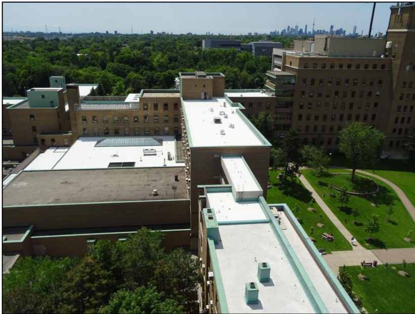
Photo 1: Multiple roof spaces at 2075 Bayview Ave - showing several retrofitted as cool roofs
