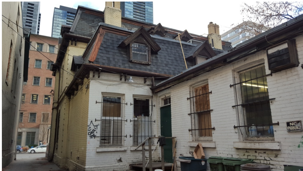
14. Current Photographs, 634 and 636 Church Street, 2016 : detailed view of the north (side) elevation of 634 Church (above) and the rear (west) walls (below) (Heritage Preservation Services).
