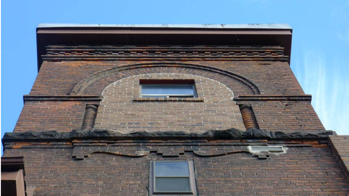
14. Tower detail, south elevation : showing the Romanesque brick checkerboard pattern, rustic stone coursing and colonettes and the Queen Anne decorative brick detail beneath the rustic stone coursing detail as well as the alterations including the bricking in of the bell tower opening and the insertion of a new window below (HPS)
