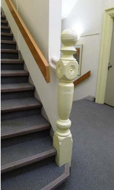
28. North Corridor : showing original stair with exposed newel post with stair handrail contained within new wall enclosure. Note also the original door case on the opposite wall. (HPS)
