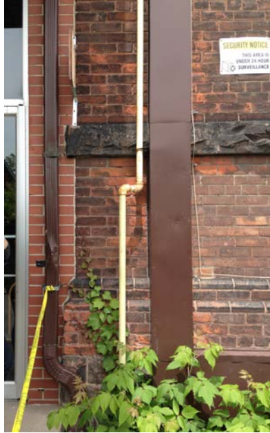
18. Junction of the Estonian House addition (left) to the Chester School (right). (HPS)
