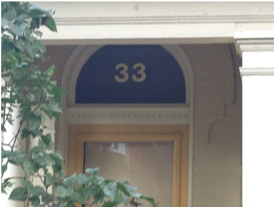
18. 33 Sussex Avenue : showing the decorative detail of the lintel over the door
