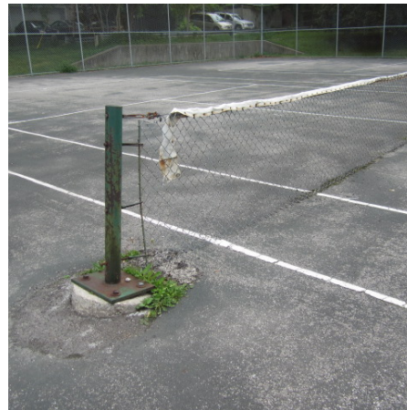
Deteriorated tennis courts
