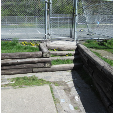
Deteriorated timber retaining walls
