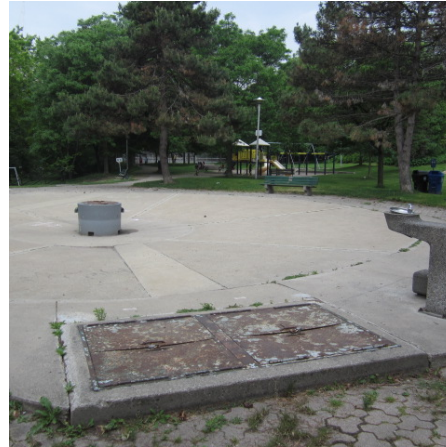
Deteriorated wading pool
