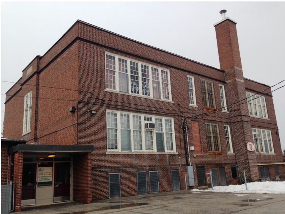
Rear (north) elevation facing the playground, showing the original double-hung wood windows and the entrance to the 1956 addition at the east side of the school (HPS, 2016)
