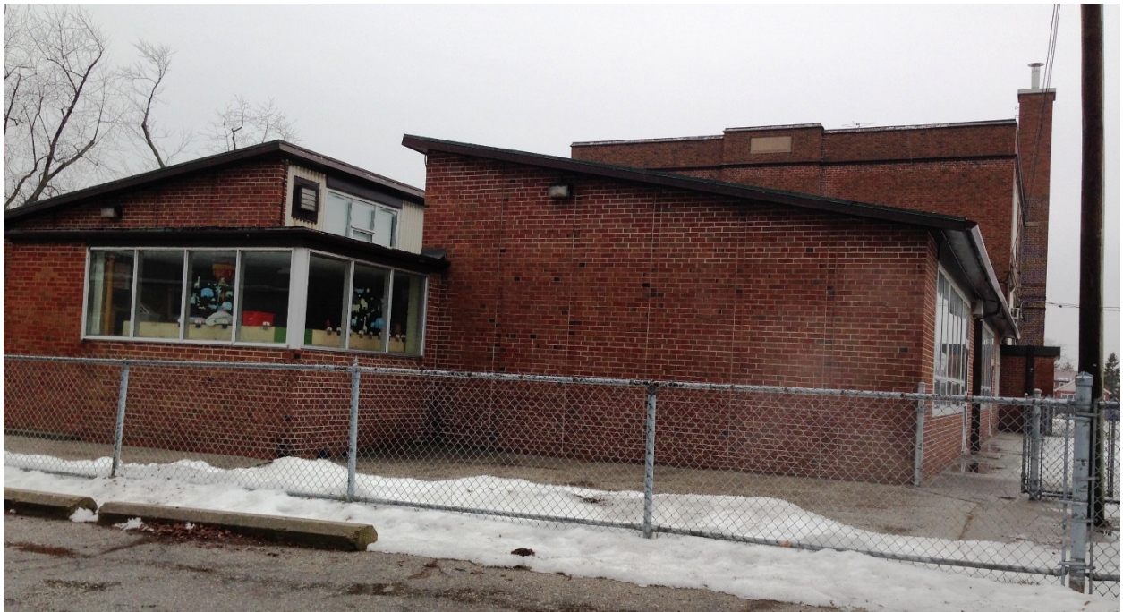
20. East addition: showing the east end with the smaller flat-roofed block with the wrap-around corner window. (HPS, 2016)
