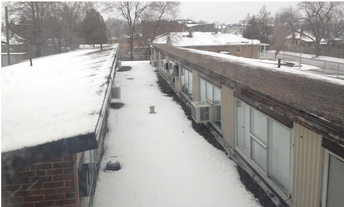
21. East addition: showing the split gable roof with the clerestory windows (HPS, 2017)
