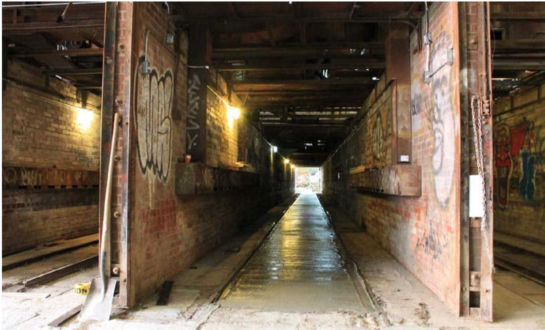
Interior of Building 16 showing the entrance to a tunnel dryer (ERA Architects Inc.)
