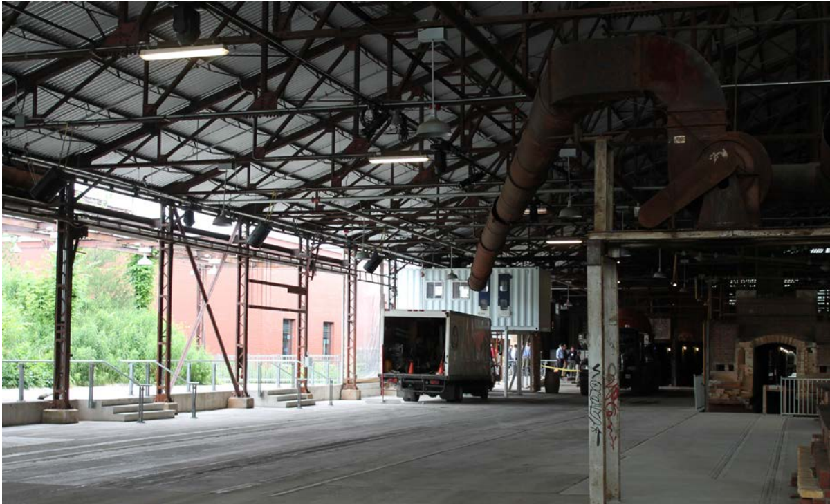
Interior of Building 16 looking north showing the open west wall (left) proposed to be enclosed with glazing, and the network of interior railway tracks embedded in the floor (ERA Architects Inc.)
