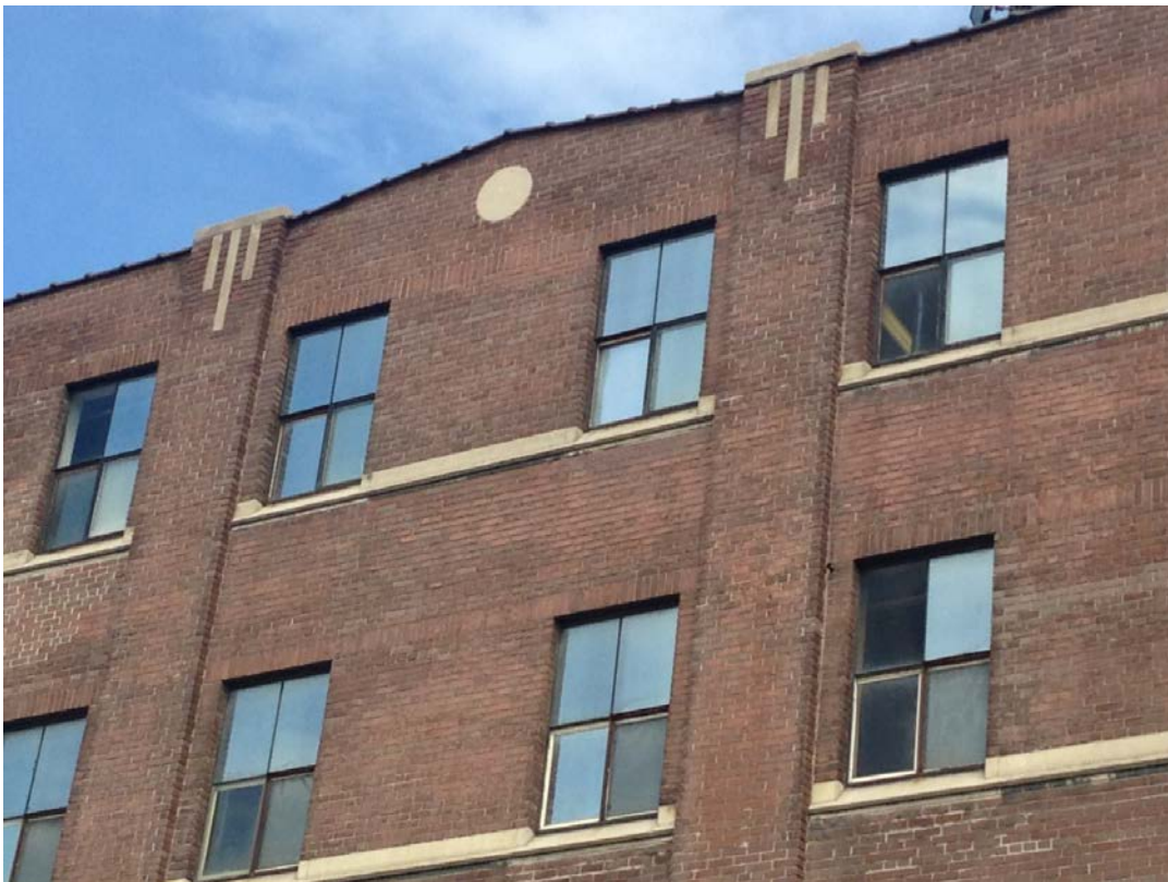
23. Principal, south elevation showing the stone details including the particular cut of the window sills, the vertical bands on the pilasters with their stone caps, the pediment with its stone disc and the vertical soldier courses above the window heads stretching from pilaster to pilaster (HPS, 2017)
