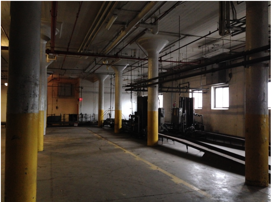
18. Interior of the east extension, ground floor showing the internal structural grid (HPS, 2016)
