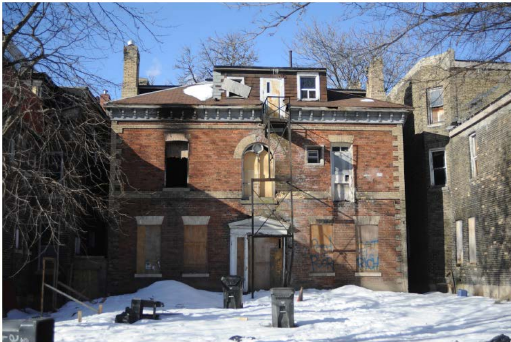
East or rear elevation of the Thomas Meredith House at 305 George Street.
