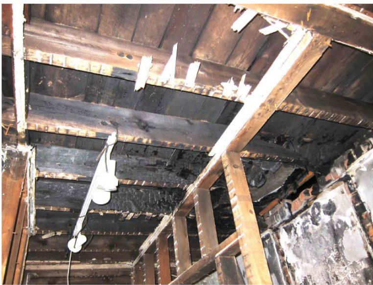
The third floor of 303 George Street (The Frank Beecroft Houses) showing evidence of fire damage
