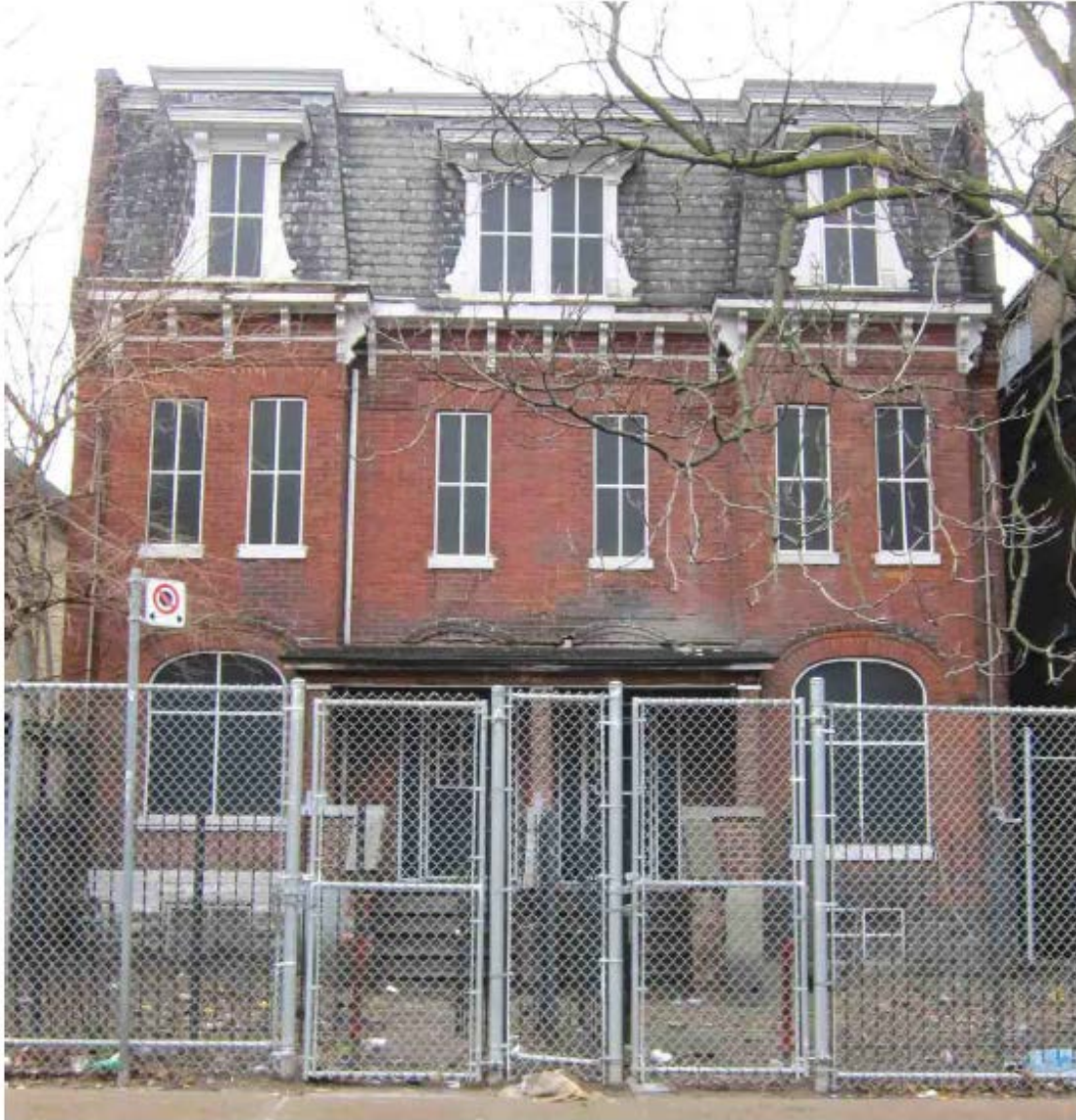
West or front elevation of the Robert Armstrong Houses at 309-311 George Street.
