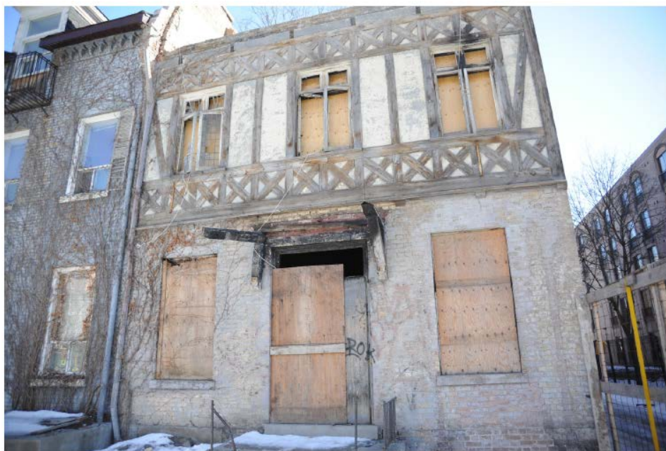
West elevation of the Fegan Boy's Home at 295 George St, shortly after acquisition by the City of Toronto
