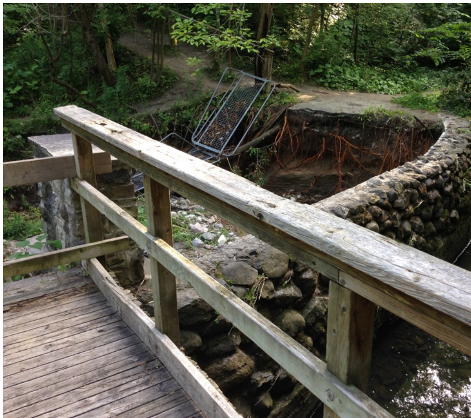
Missing path to southern bridge (stream to right of wall, washout to left)
