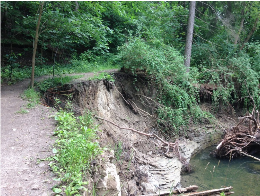
Washout on eastern footpath (as of early August)
