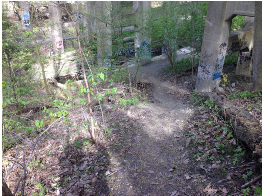
Foot-eroded steep footpath down to stream by railway bridge
