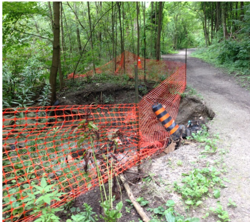
Growing washout at northern footbridge
