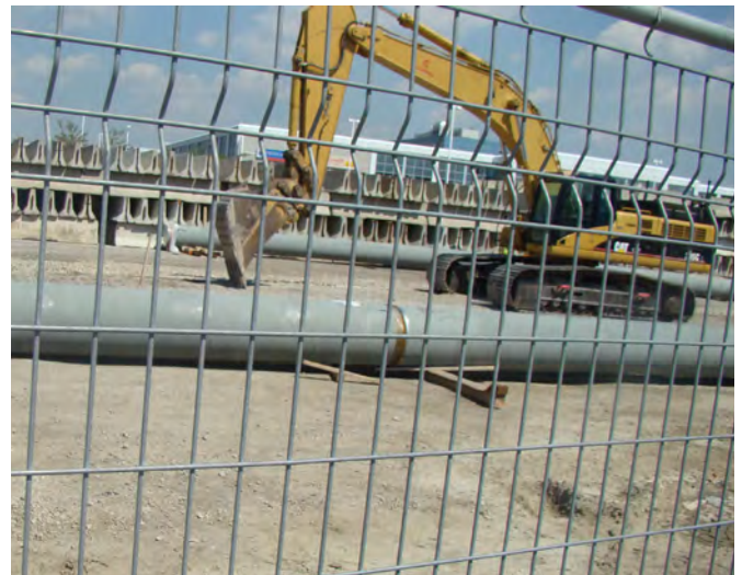
Figure 49: Some watermains will be relocated and replaced through construction of the LRT portal
