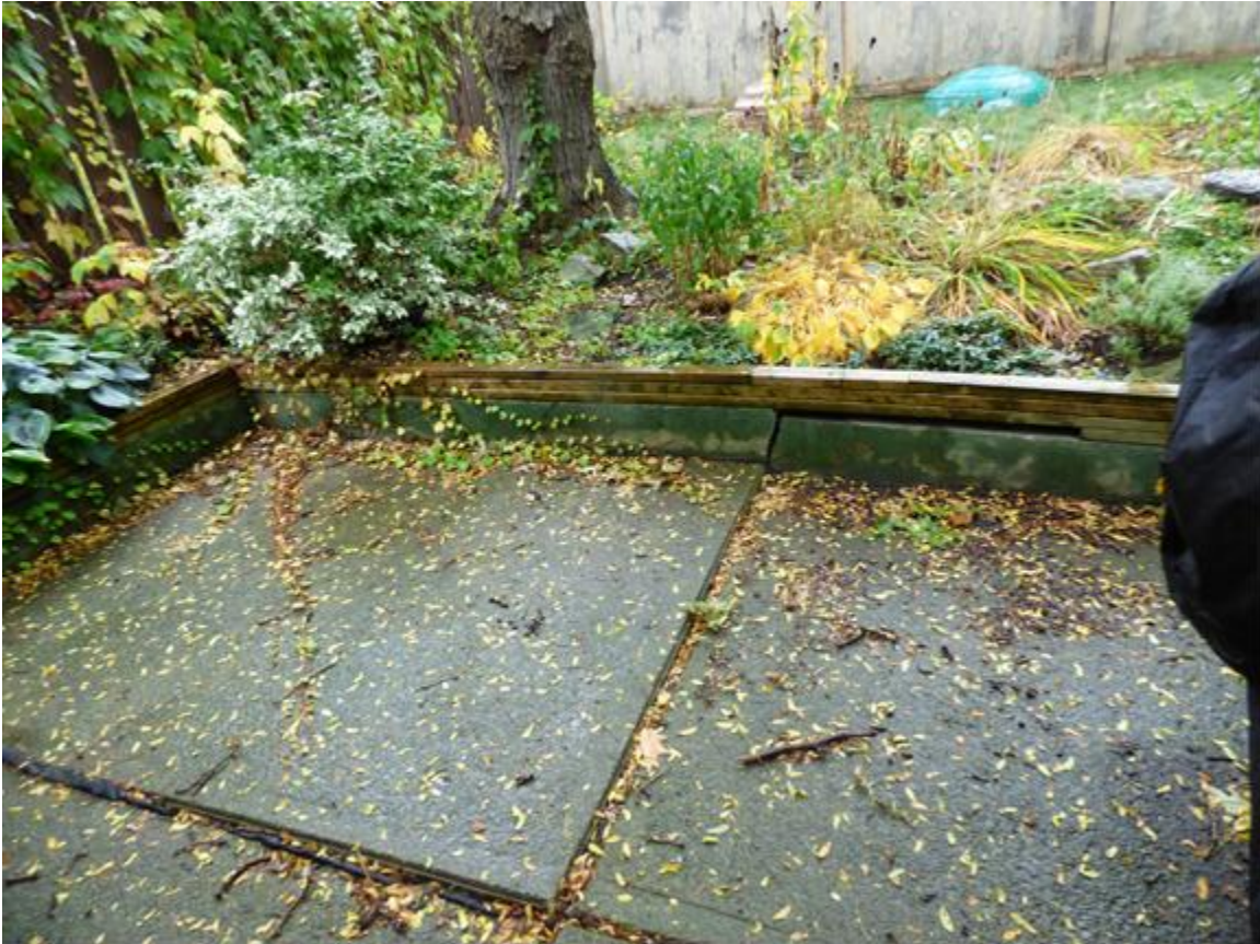
Attachment 2 – Photograph showing cracked retaining wall and lifted concrete slab.
