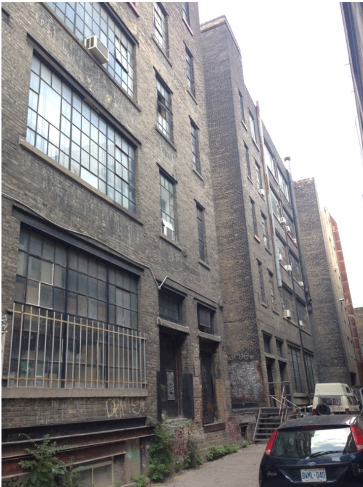
24. Rear (south) elevation, showing the original steel window sash, arrangement of openings and original delivery doors (HPS, 2017)
