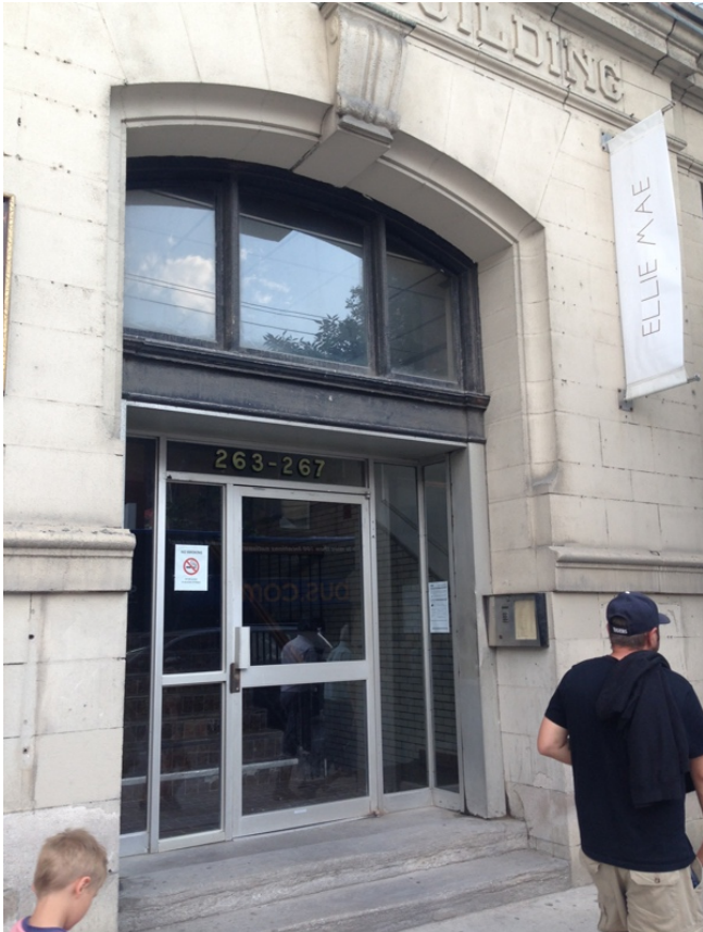
19. View of the entry with the stone surround, transom light and later doors (HPS, 2017)
