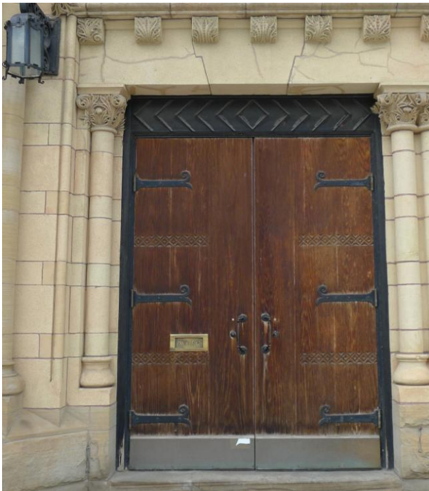
29. 115 Bond Street: showing the left-hand pair of the new set of doors installed prior to the 1980s renovations (HPS, 2016)
