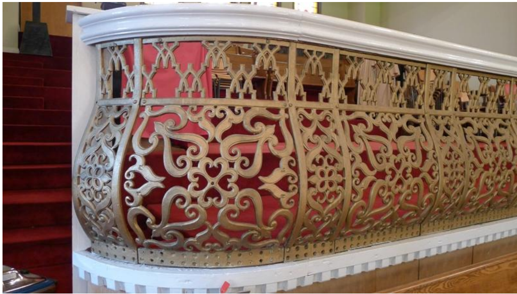
35. 115 Bond Street, Balustrade: showing the gallery balustrade composed of pressed metal panels in an arabesque design. (HPS, 2016)
