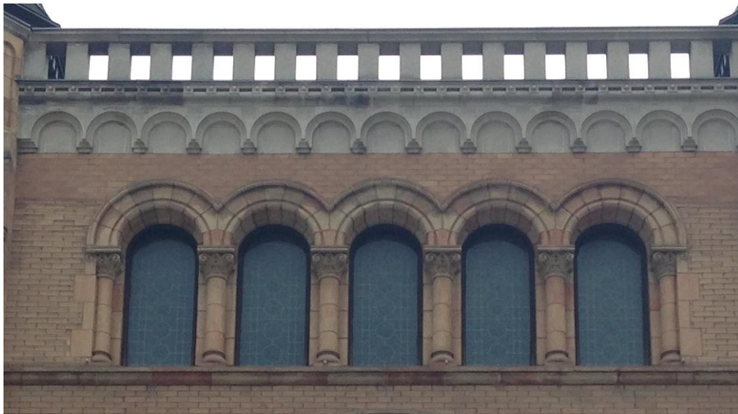
26. 115 Bond Street: showing the arcade at the third level above the tympanum with its row of colonettes and composite capitals and above the restored parapet of arches and balustrade (HPS, 2016)
