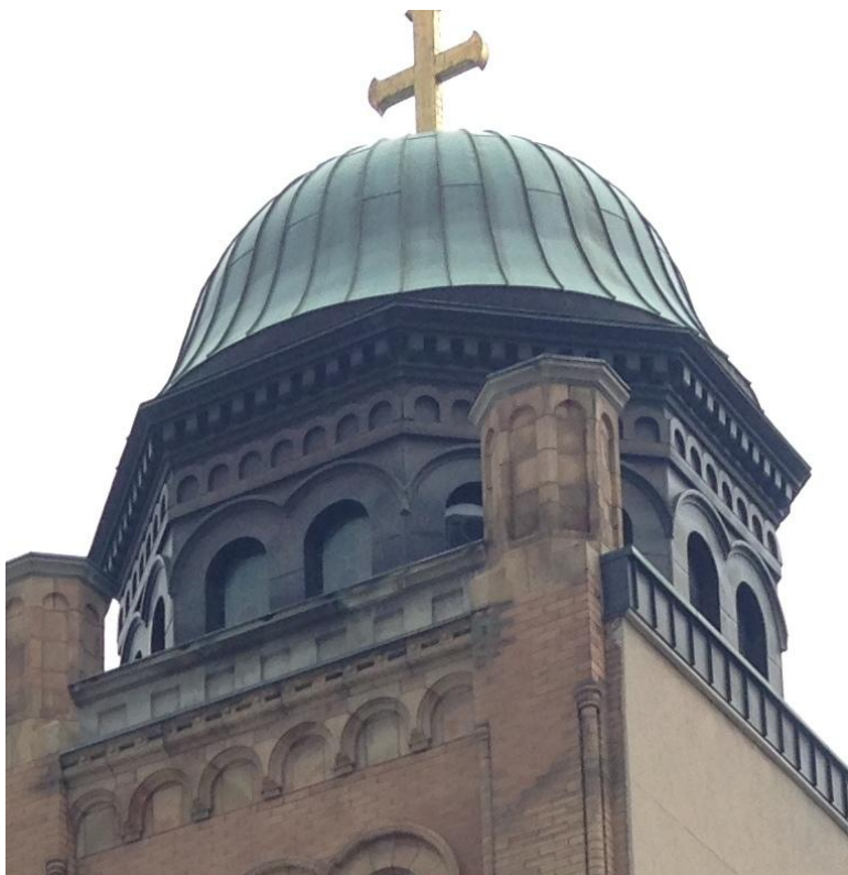
27. 115 Bond Street: showing one of two original octagonal drums on the towers with its richly detailed cornice and pairs of windows, as well as the octagonal turrets terminating the piers of the tower. Note the arches of the parapets and the brick colonettes with their capitals. The new copper dome with its bell cast curve and the cross were part of the 1980s renovations (HPS, 2016)
