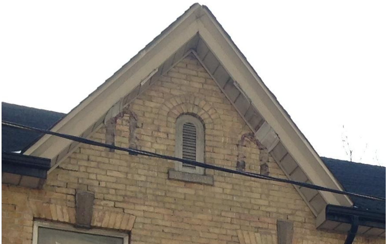
25. 81 Shuter Street, North elevation, gable detail: showing location of former wood brackets. (HPS, 2016)
