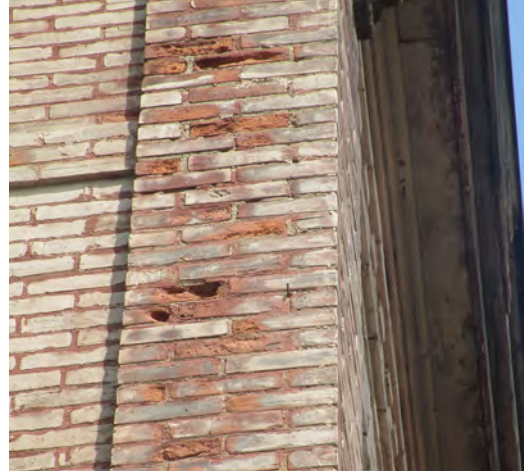
Fig.21: Spalled bricks at corner of building, South elevation.
