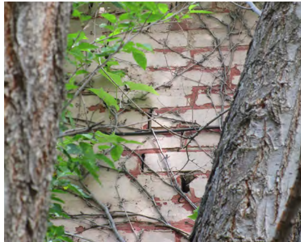
Fig.23: Cracked bricks and open mortar joints, South elevation.
