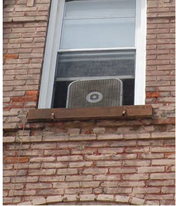
Fig.5: Spalled bricks at either side of window, and underneath sill. Parge repairs to bricks underneath sill
