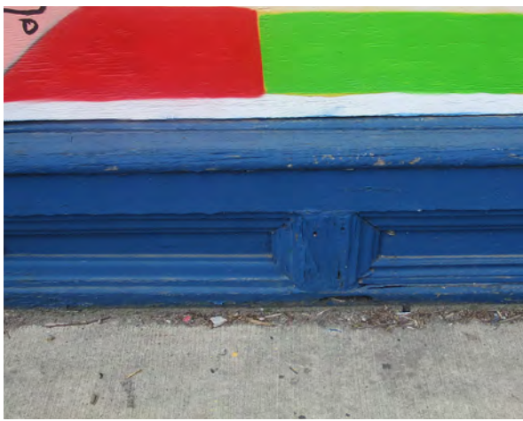
Fig.13: Weathered paint at base of window frame, East elevation.
