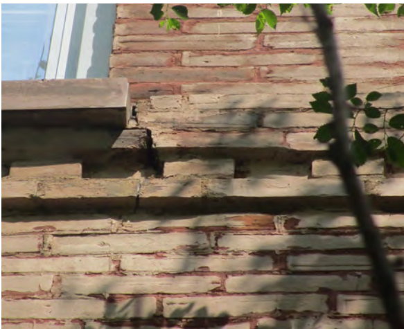
Fig.24: Patching repair to bricks, and open mortar joints adjacent to sill, South elevation.
