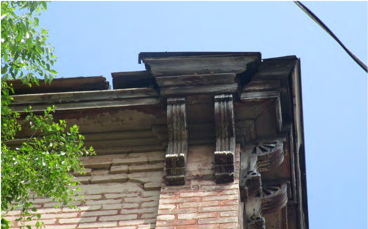
Fig.40: Poor condition of cornice, out of alignment, with holes and pieces missing.
