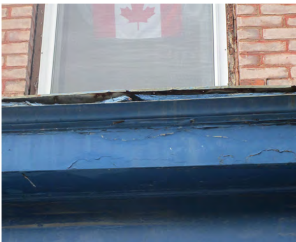
Fig.12: Poor condition of flashing to cornice above window, East elevation.
