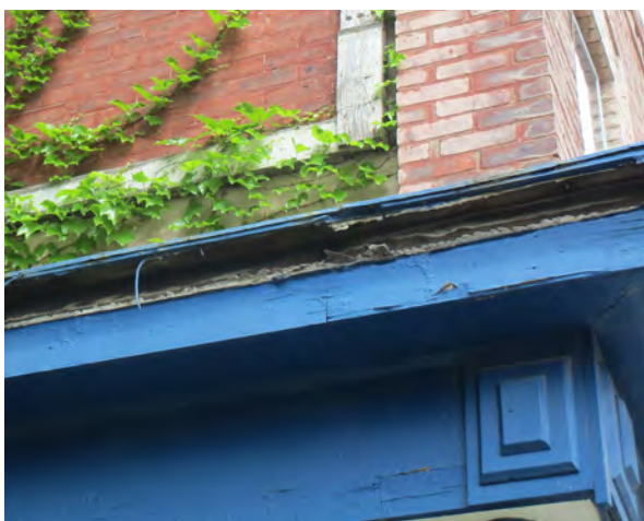
Fig.37: Poor condition of cornice with piece missing at South elevation.
