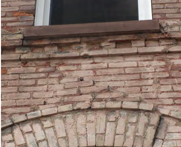
Fig.8: Cracked arch protruding and out of alignment. Parge repairs to spalled bricks underneath sill, East elevation.
