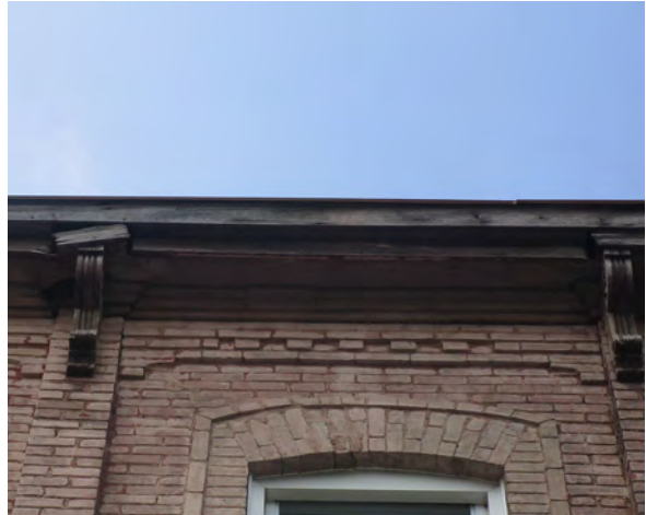
Fig.15: Weathered cornice, and slipped timber pieces above bracket, East elevation.
