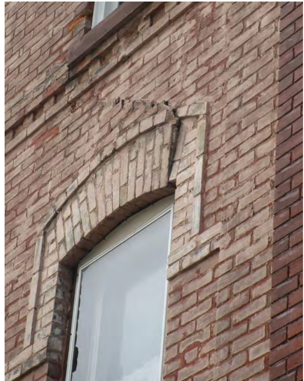
Fig.7: Cracked bricks, and defective arch protruding from building, East elevation.
