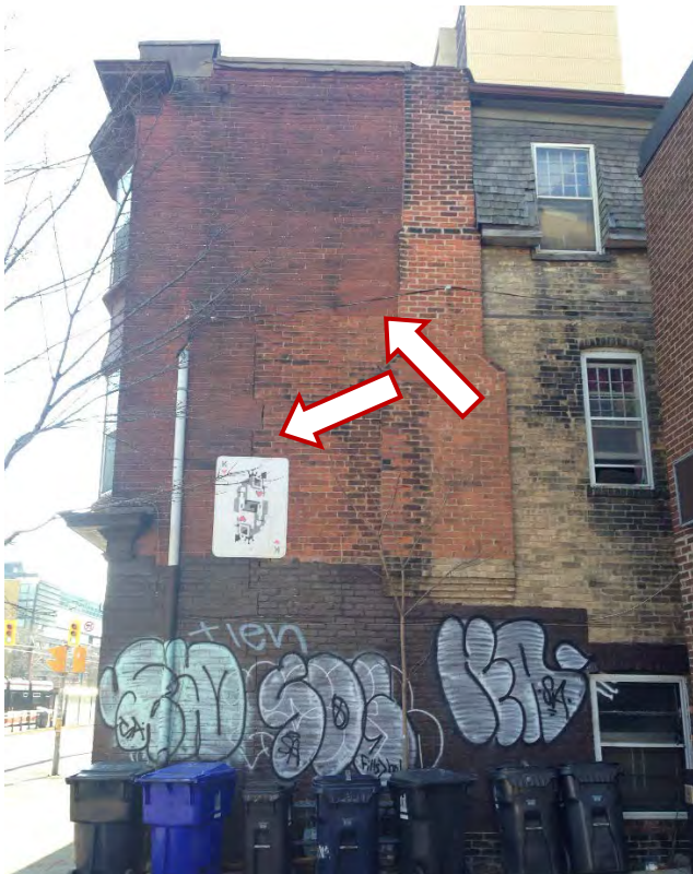
10. Photograph of the north (side) elevation of 700 Spadina Avenue showing the difference in brick and the keying of new brick with old at the left indicating the extension of the building to the east and the addition of the third storey between 1924 and 1945. (HPS, 2017)
