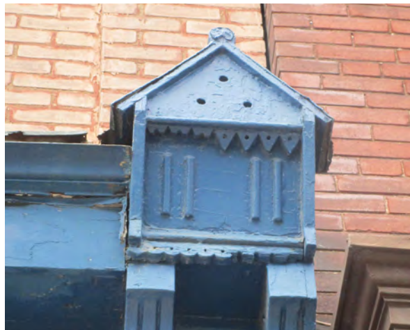
Fig.11: Pediment missing decorative details, East elevation.
