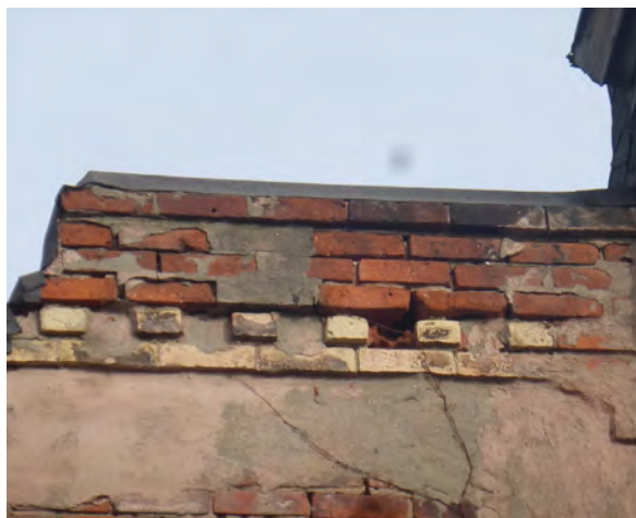
Fig.30: Poor condition of partial parapet wall, with open mortar joints and hole in brick at South elevation.
