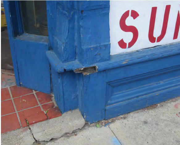
Fig.14: Hole in window frame, East elevation.
