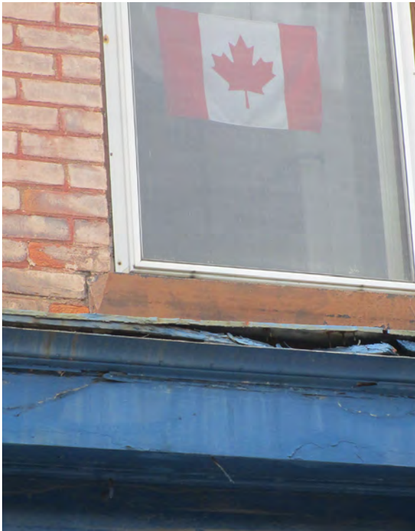
Fig.6: Chip in sill, and spalled brick adjacent to sill, East elevation.
