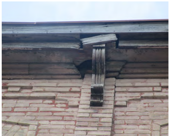
Fig.17: Holes in soffit. Note weathered bracket that appears to be in a fair condition, East elevation.
