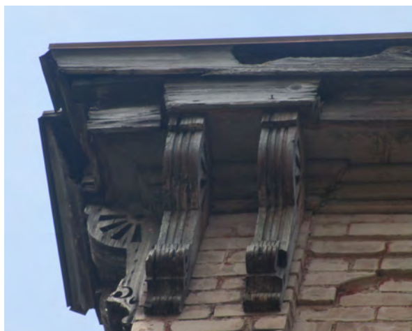
Fig.19: Holes in cornice and soffit, East elevation.
