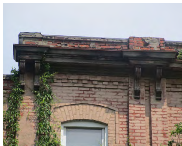
Fig.31: Poor condition of parapet wall, with spalled bricks at South south elevation.
