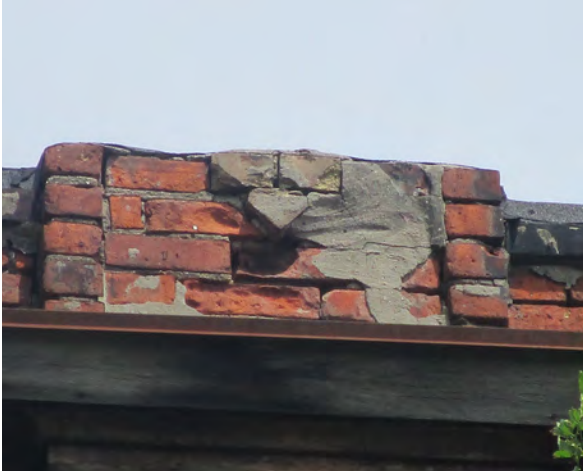
Fig.32: Poor condition of parapet wall, with spalled bricks, parged repair, and open mortar joints at South elevation.
