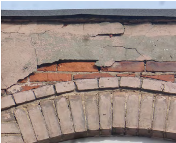
Fig.28: Cracked parging at third floor, with spalled bricks below, and open mortar joints at South elevation.
