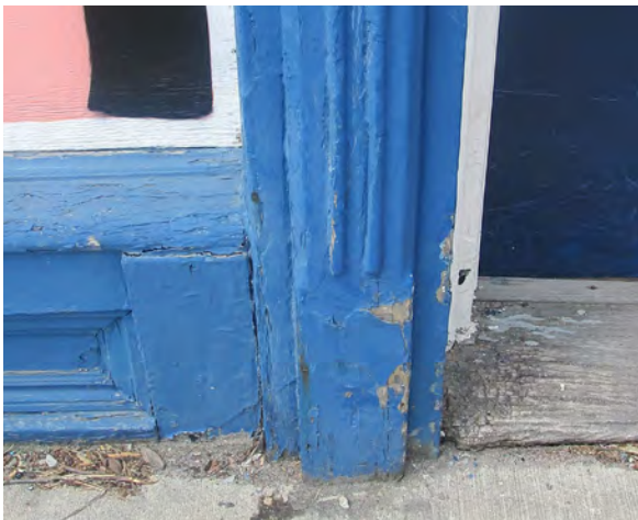
Fig.10: Weathered and peeling paint from window frame on East elevation.
