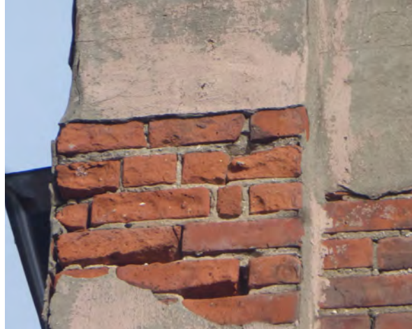
Fig.33: Spalled bricks and open mortar joints at third floor at South elevation.
