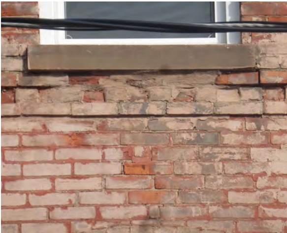
Fig.34: Parged bricks below window sill at South elevation. Note open mortar joints, and spalled bricks.
