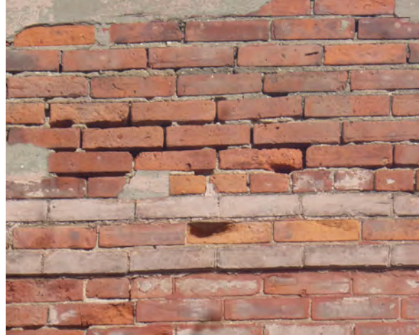
Fig.27: Spalled bricks and open mortar joints at third floor of South elevation.
