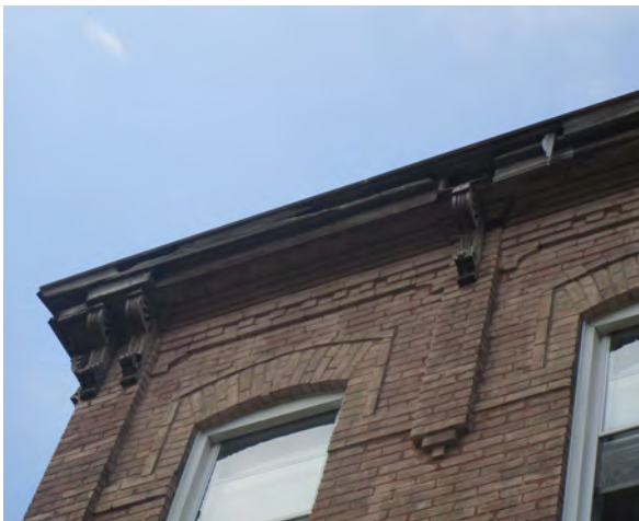
Fig.16: Holes in cornice and soffit, East elevation.
