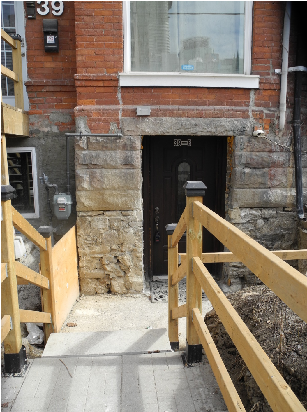
19. Photograph showing new stair and excavation of the footings at 39 Mutual Street to replace the original window opening with a door (CBCollective, 2018).
