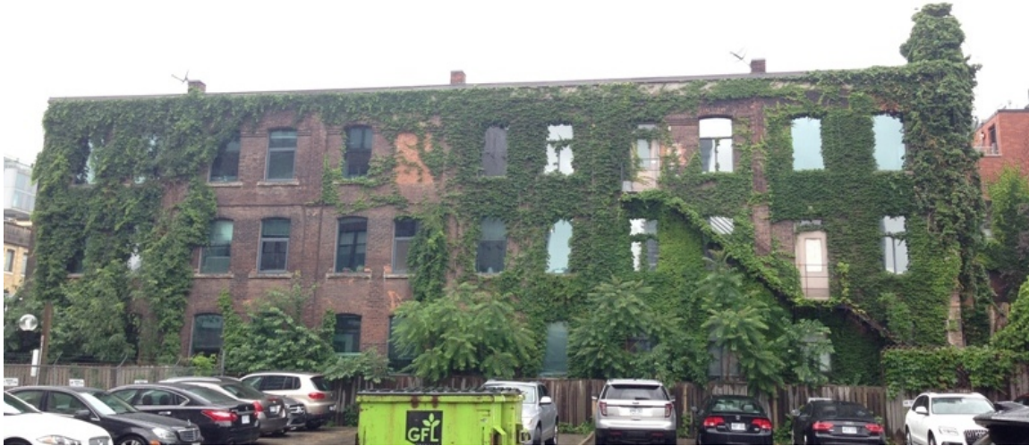
13. South Elevation showing the original brick colour and the fire escapes. (HPS, 2018)
