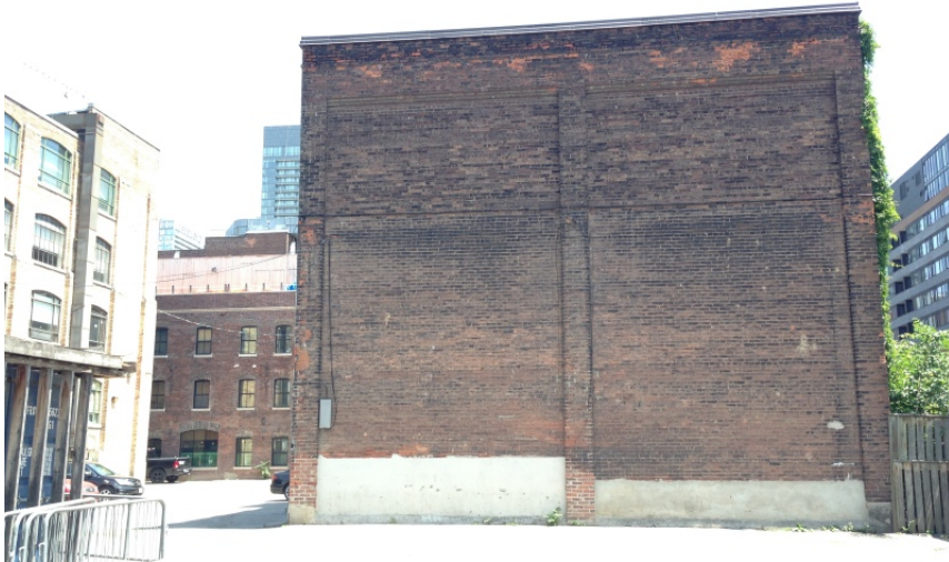
14. West elevation showing the two structural piers of the end wall and the absence of openings (HPS, 2018)
