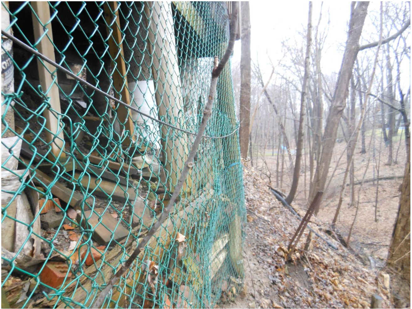
Photo 5. Photograph of the area below the existing deck in relation to ravine. Photo taken March 07, 2017 by RNFP Staff.
