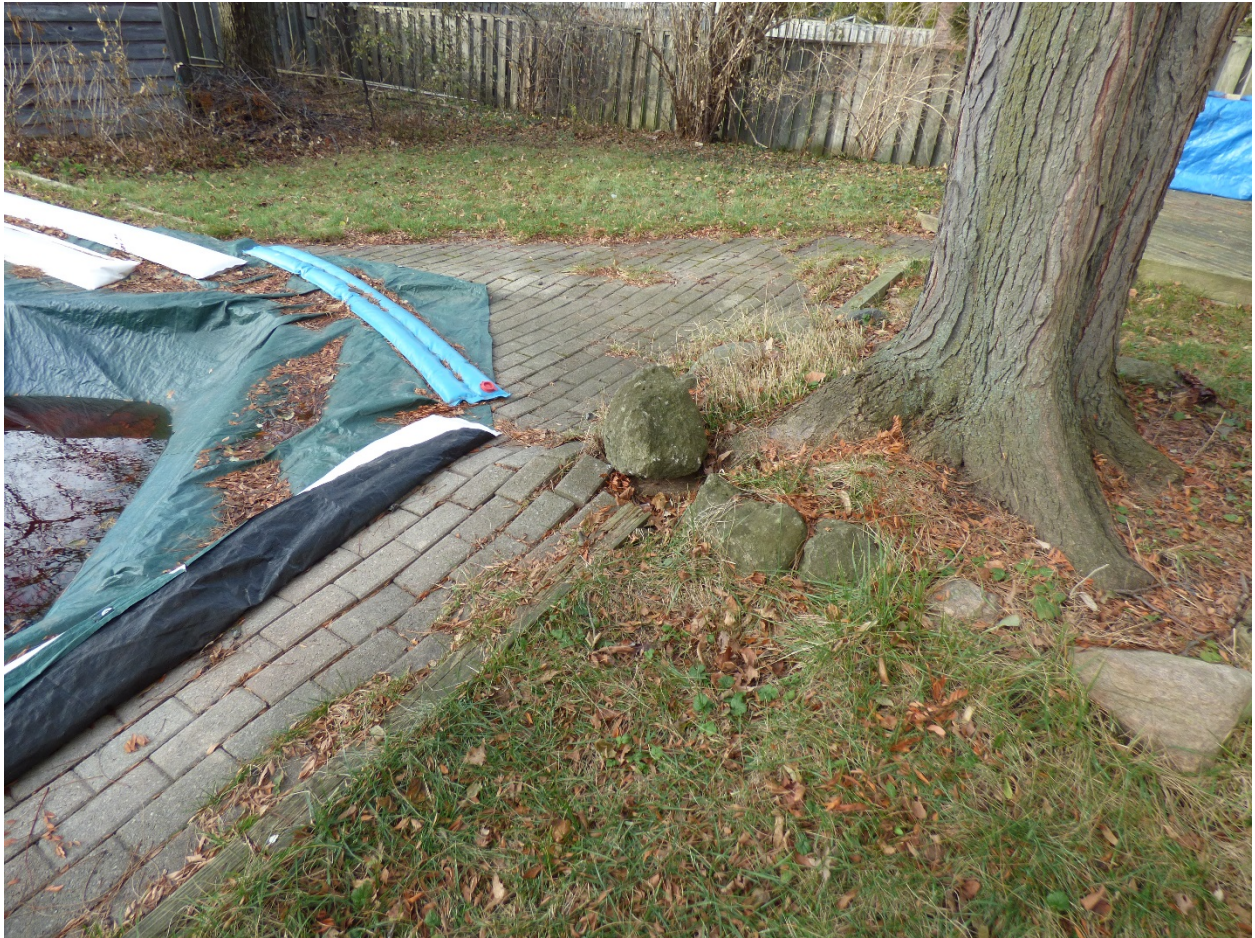
Attachment 2 - Photograph of the pool and interlocking brick at the base of the honey locust tree measuring 68 cm in diameter
