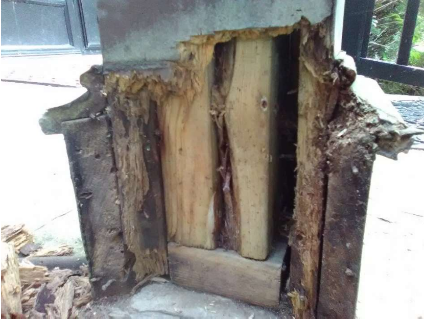
Figure 1 : Modern Wood Framing of Porch Column incorrectly cited as a Heritage Attribute
