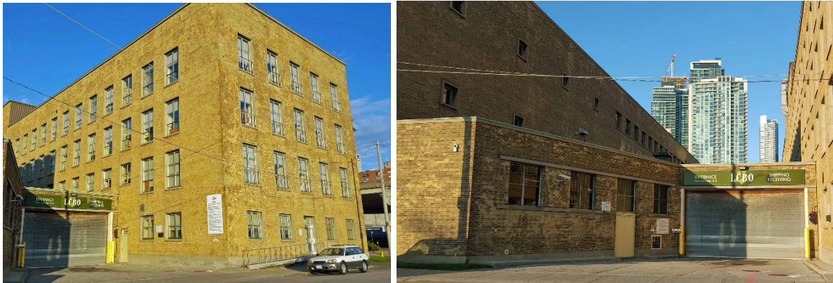
5d and 5e. Office Building, showing the east elevation and part of south elevation (left), and the enclosed link between the office building and the warehouse from east (right)
