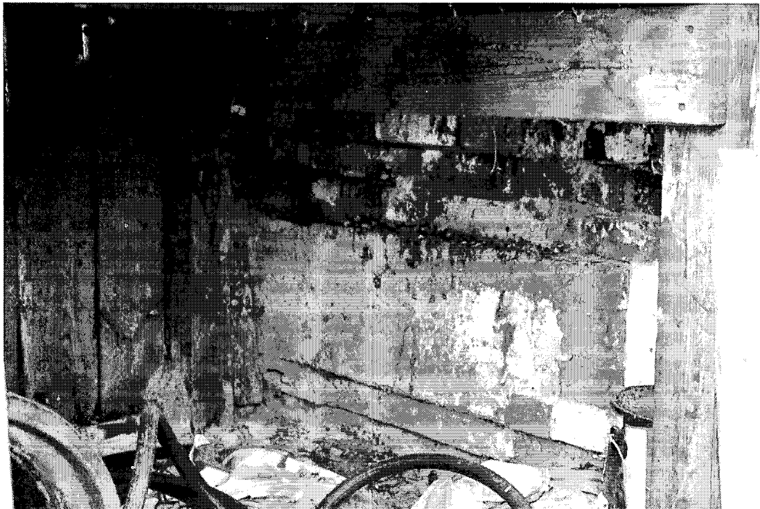
Figure 4: West facade of Jefferson Ave located south of the Liberty Village Market and Cafe entrance steps. The exposed painted brick wall is present under wood framed storage areas on the north and south sides of the steps.
