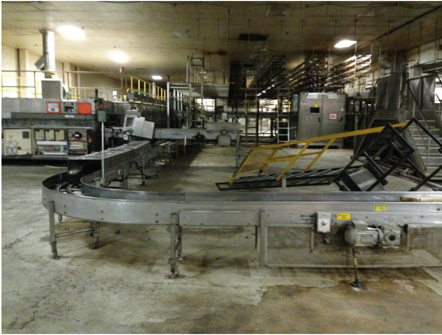
19. Interior of one of the rear additions showing remaining bakery machinery (HPS, 2016)
