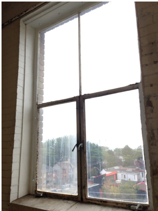
16. Interior view of metal windows installed with the 1926 additions to the complex, showing the opening bottom sections.
