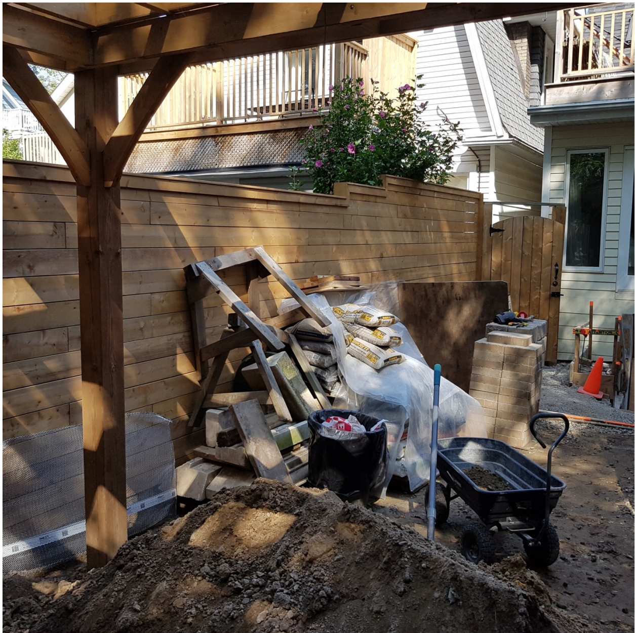
Attachment 2: Existing fence on West side of property (photo taken facing North)
