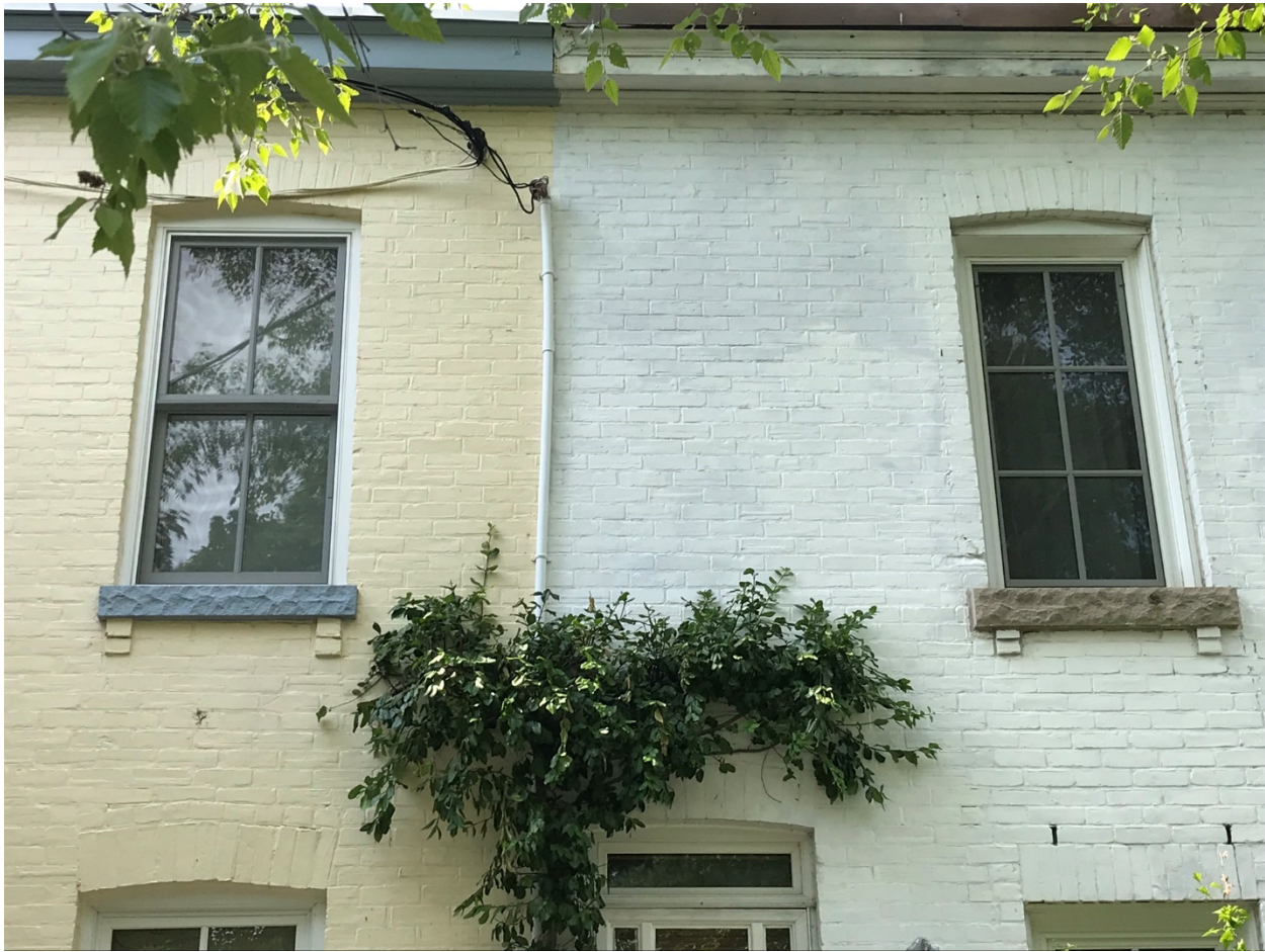
10. Photograph showing the window opening detailing with the rough-cut stone sills supported by brick corbels (HPS, 2018)
