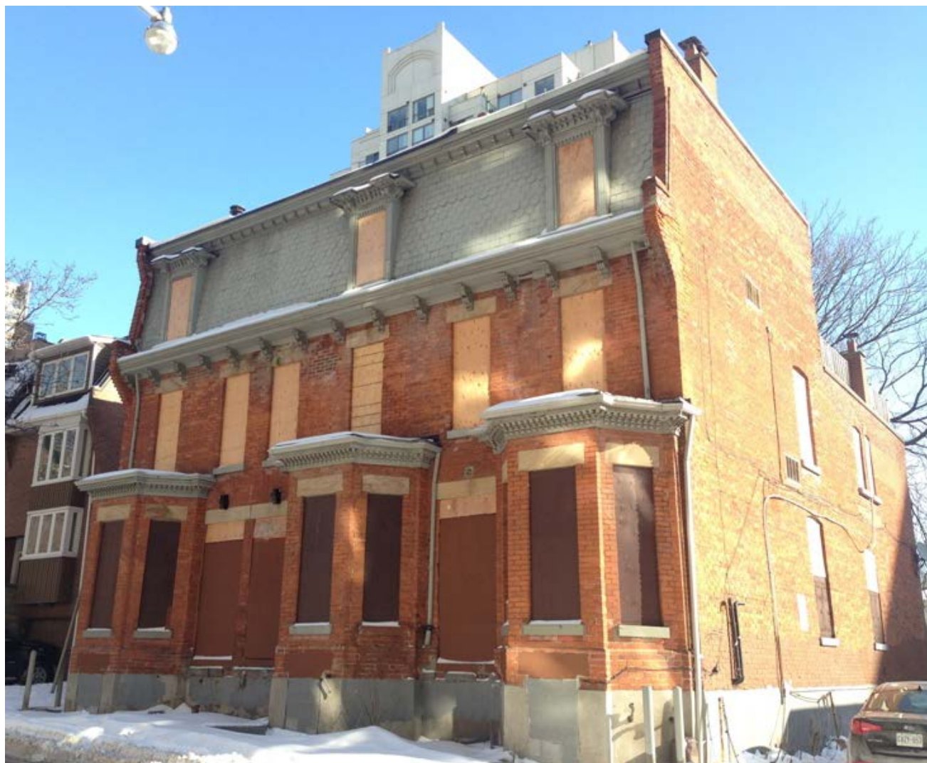
2019 photograph of the heritage properties at 189-193 Mutual Street, the Mutual Street row houses which were designated in 2015 under Part IV of the Ontario Heritage Act under By-law 1294-2015. This photograph shows the condition of the properties following the fire.
