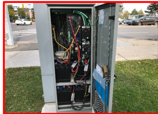
Figure 8: Inside the UPS
