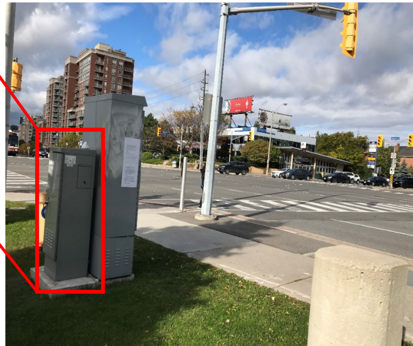
Figure 7: A UPS installed at a signalized intersection
