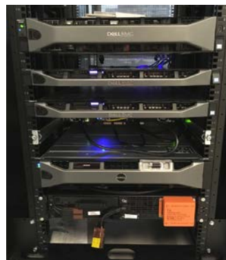
Figure 15: SCATS Smart Traffic Signal Control System Installation
