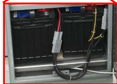
Figure 9: The UPS batteries
