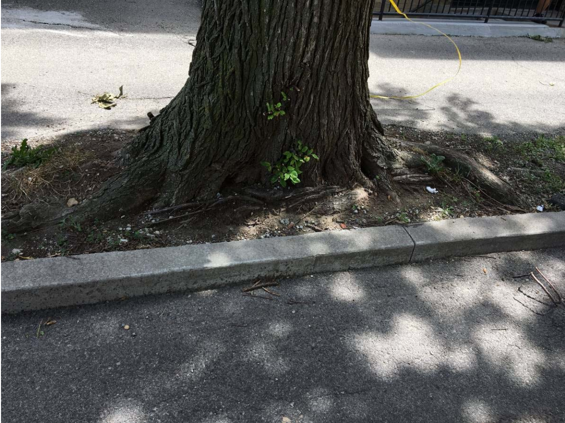
Attachment 4 – Photograph of the subject tree's trunk flair from the west looking east, showing the 160 Erskine Avenue driveway
