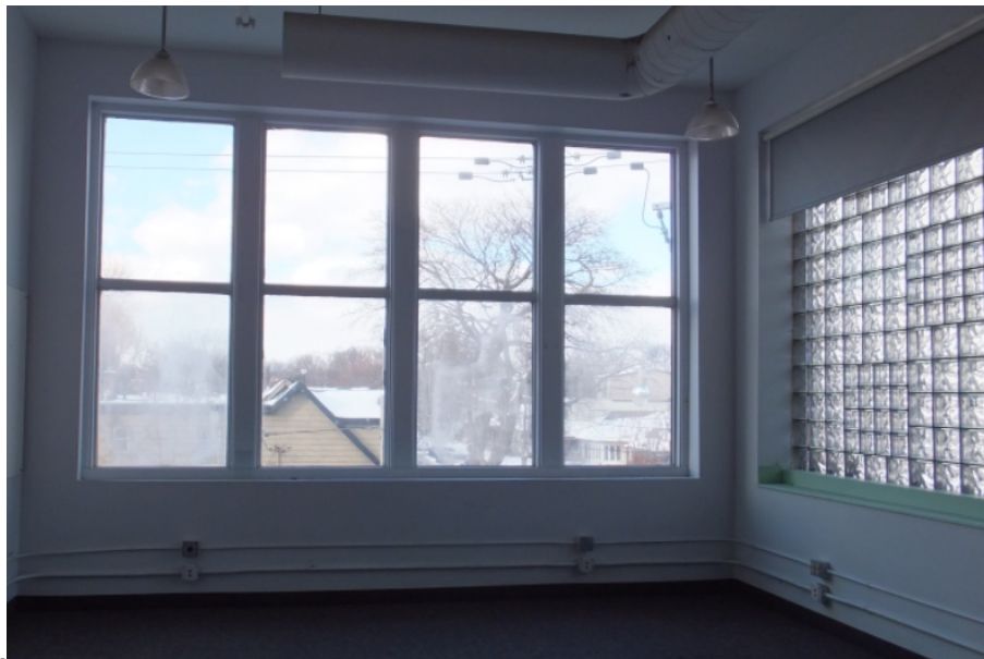
43. Main Building (A), Interior, Second Floor showing the north and east elevations with glass block (HPS, 2018)
