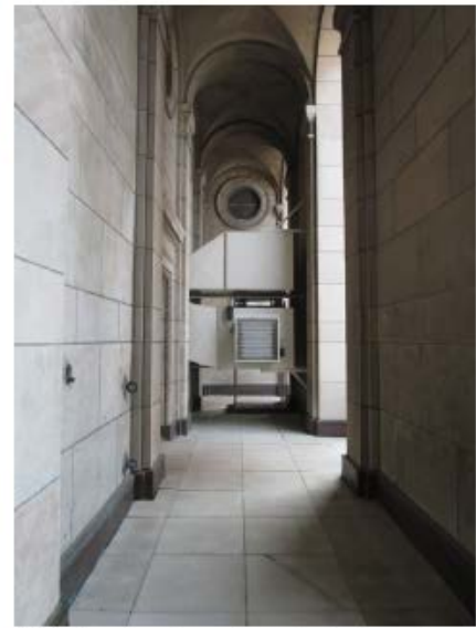
32 nd floor loggia and mechanical equipment (ERA, 2017).
