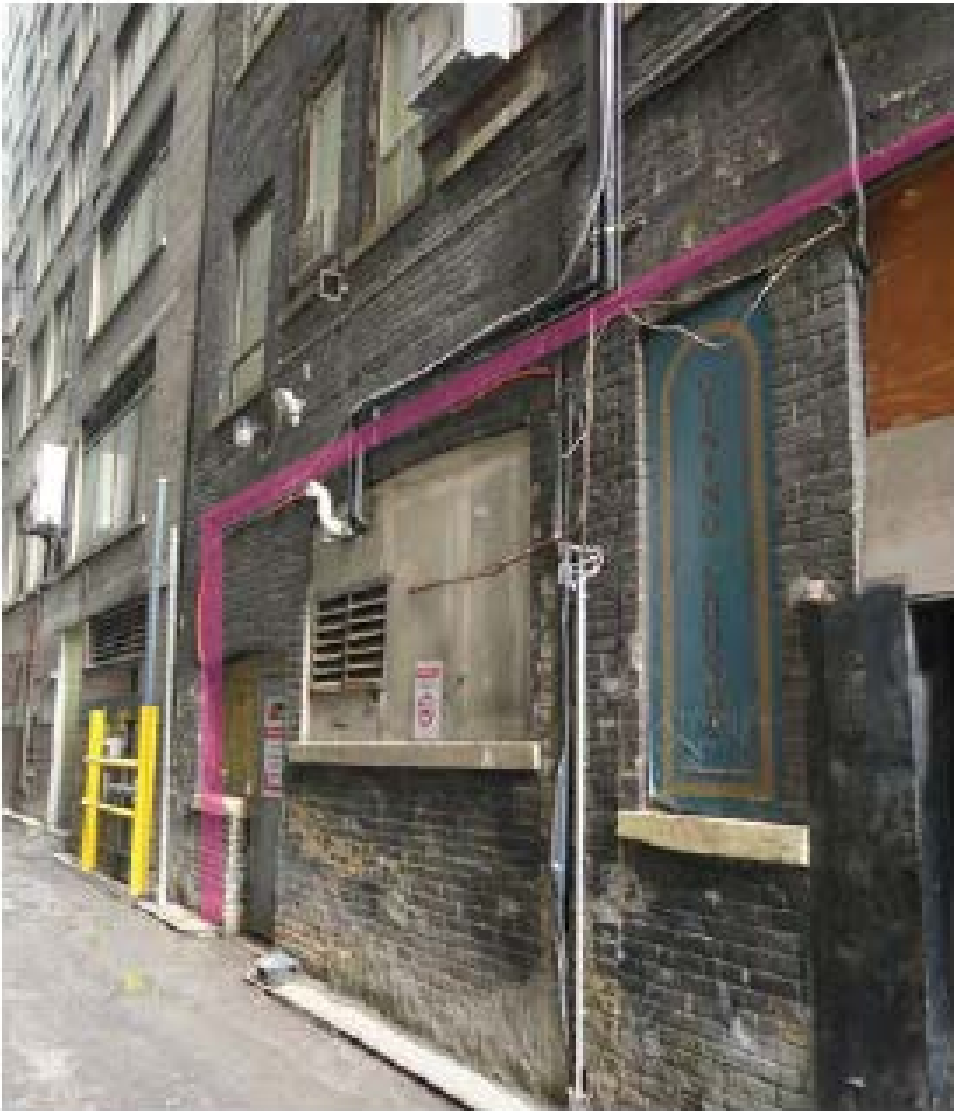
Rear (west) elevation of 56 Yonge from laneway; pink line denotes zone below concrete sill (ERA, 2019).
