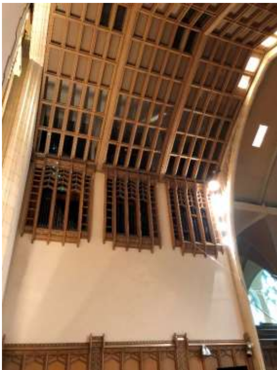
41. View of the new ceiling in the choir with openings for the organ pipes (HPS, 2019)
