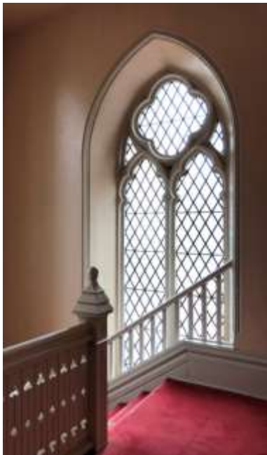
45. View of the window in the east stair tower, repaired following the fire in 1954 (HPS, 2019)
