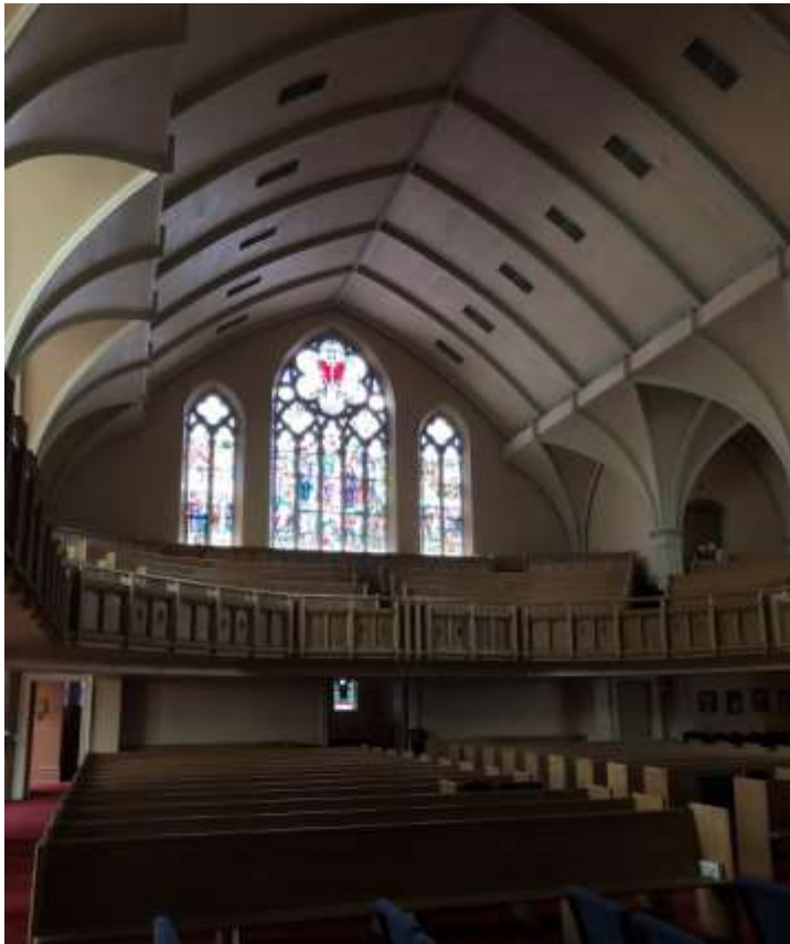
42. Interior looking south showing the new structure of the columns, arches and ceiling (HPS, 2019)
