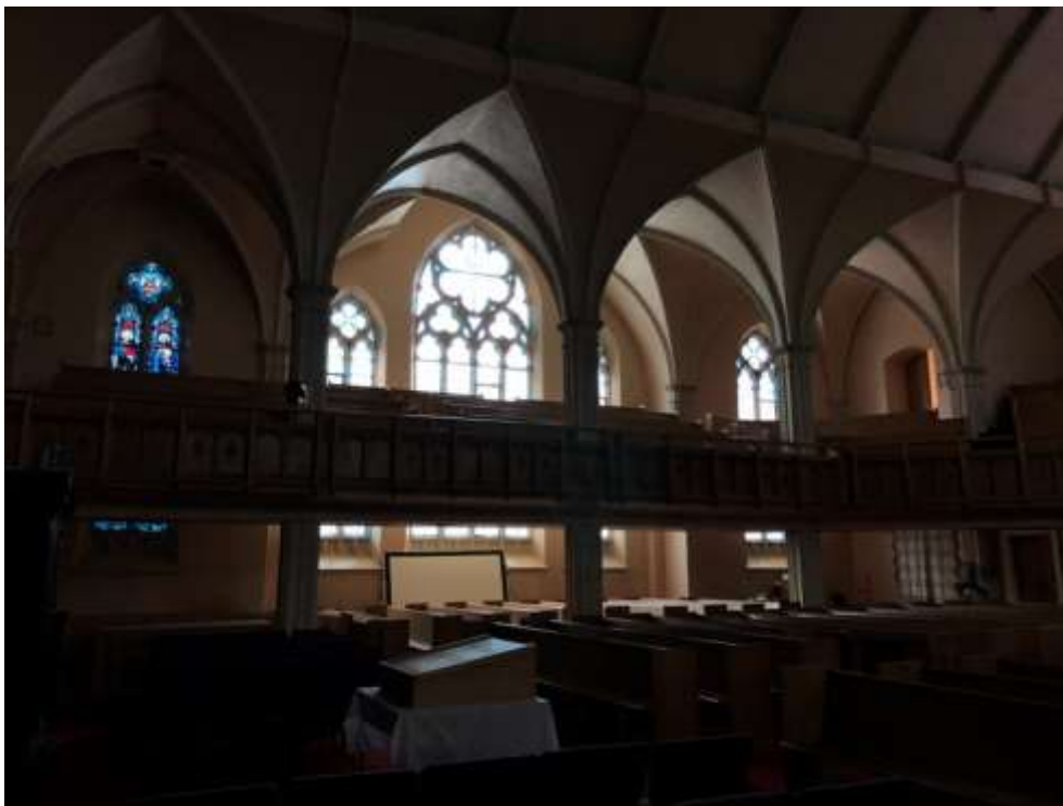
43. View of the new 1954-5 structure looking to the east elevation where side aisles are created by the arches over the galleries (HPS, 2019)
