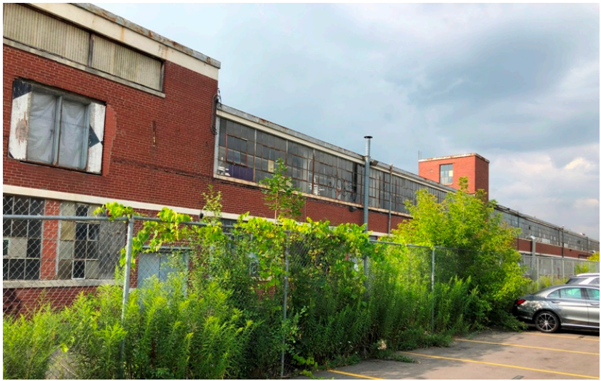
North elevation showing the raised east end and elevator towers in contrast to the horizontal ribbon windows of factory sash glazing (HPS, 2019)
