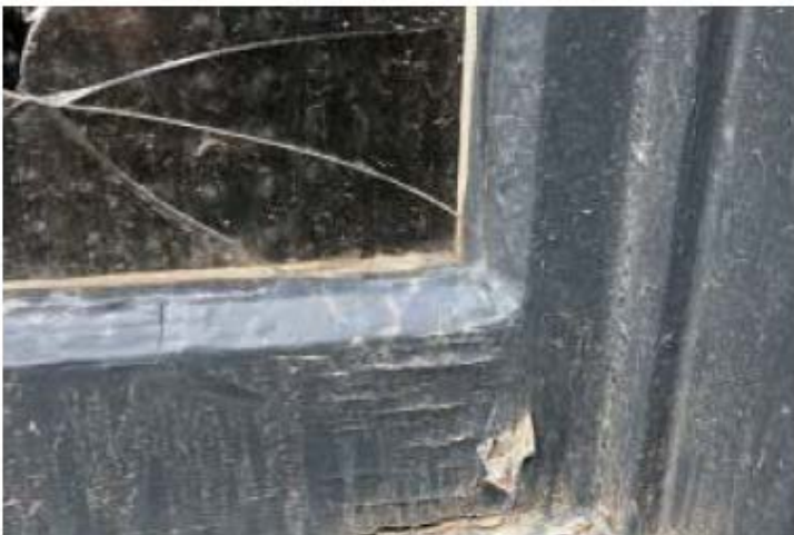
Broken glass pane & peeling paint
