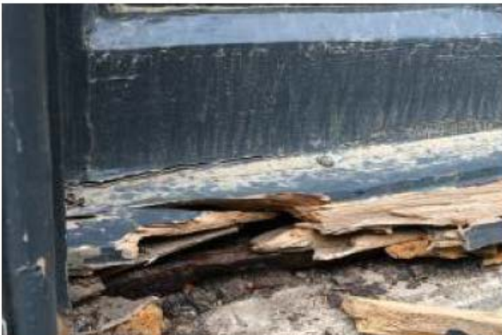
Broken sill, rusted substructure
