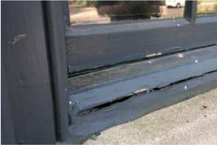
Heaved and split window sill
