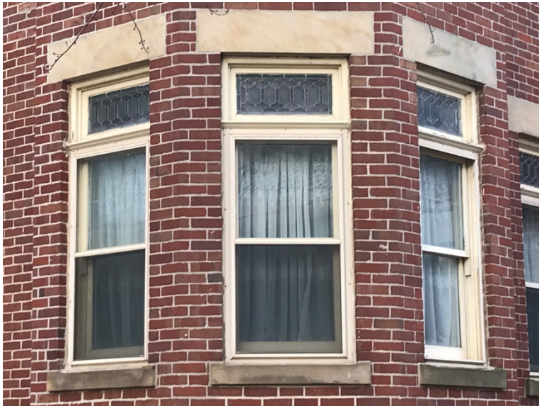
11. Image showing the decorative glass transoms above the double-hung sash windows at the first-floor level on the corner tower (Heritage Preservation Services, 2018)
