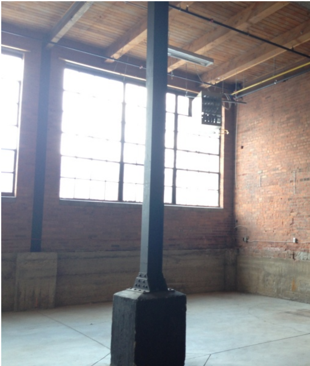
44. Main Building (A), Ground Floor, showing the grid of structural steel columns and the integration of the columns within the exterior walls (HPS, 2018)
