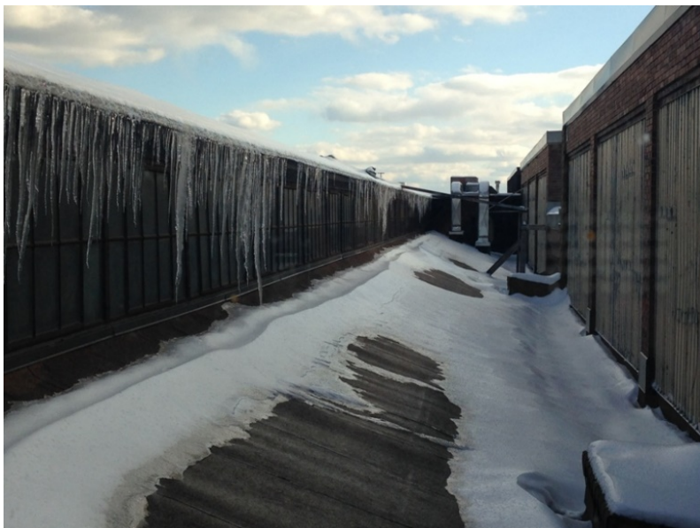
22. Building G showing the clerestory roof, left. On the right are the upper levels of Main Building (B + C) (HPS 2018)
