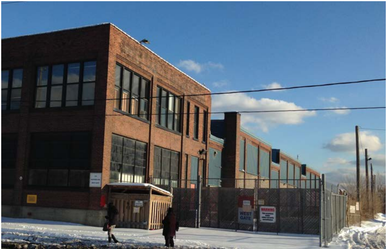
18. Side (west) Elevation viewed from Eastern Avenue of the Main Building (A B + C) showing A, the front building, B, with the chimney and two bays, and C, the later addition, with the single bay at the back of the site. The original glazing of B + C has been concealed (HPS, 2018)
