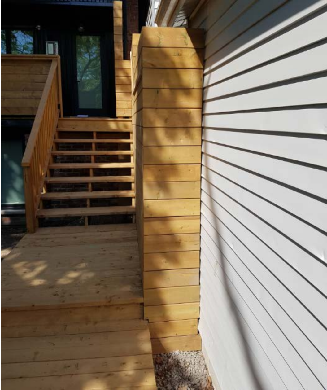
Small section of the existing fence located at the bottom of the stairs measuring approximately 1ft wide
