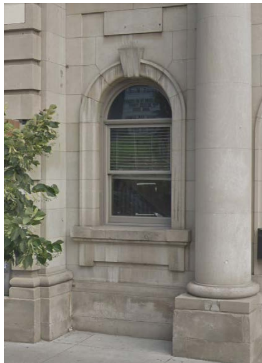
Image (facing north) of the ground floor west window to be converted to a door entrance
