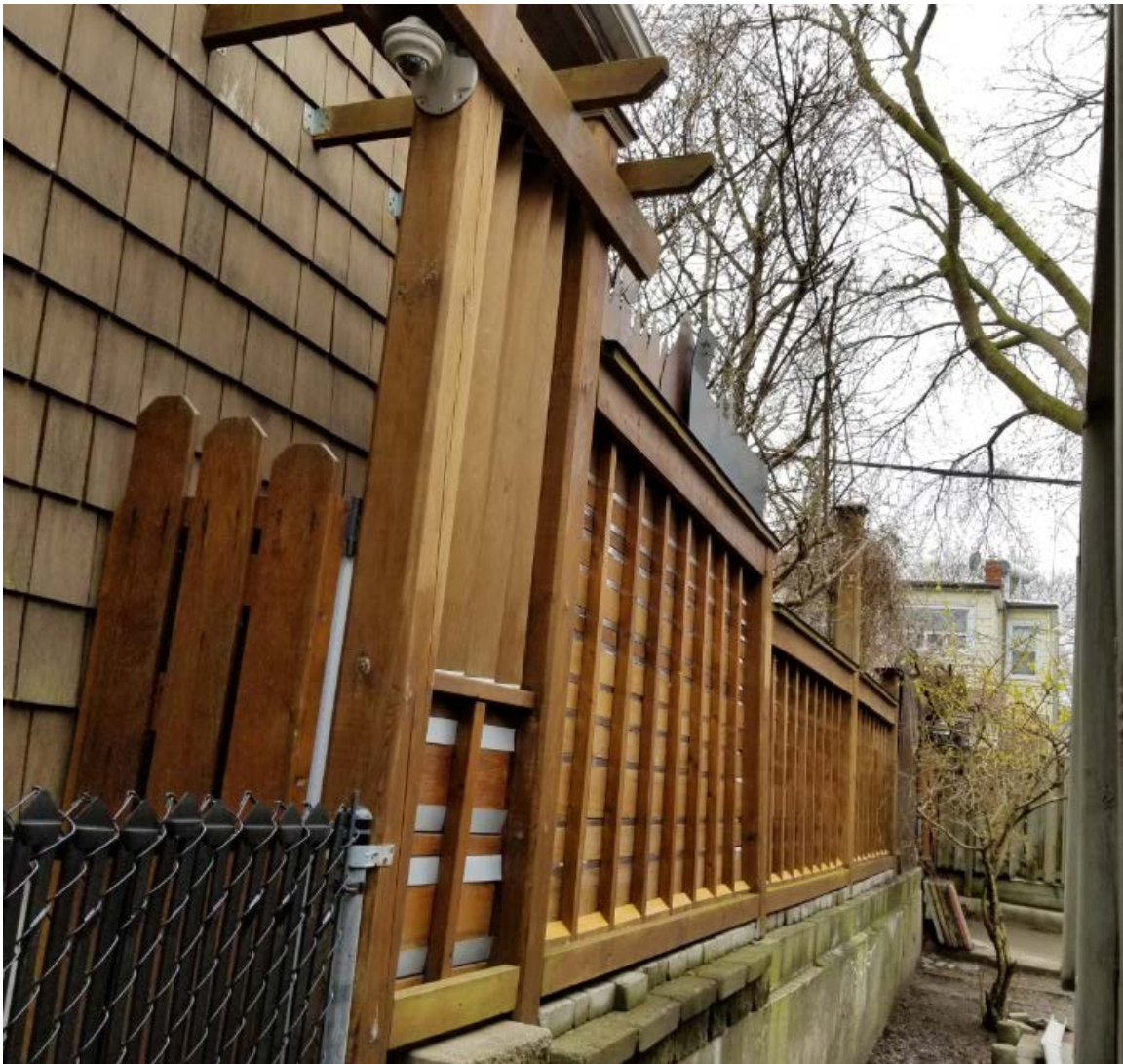
Retaining wall measures 1.04 metres, with a 2.37 metre high wooden fence panel attached on top.
