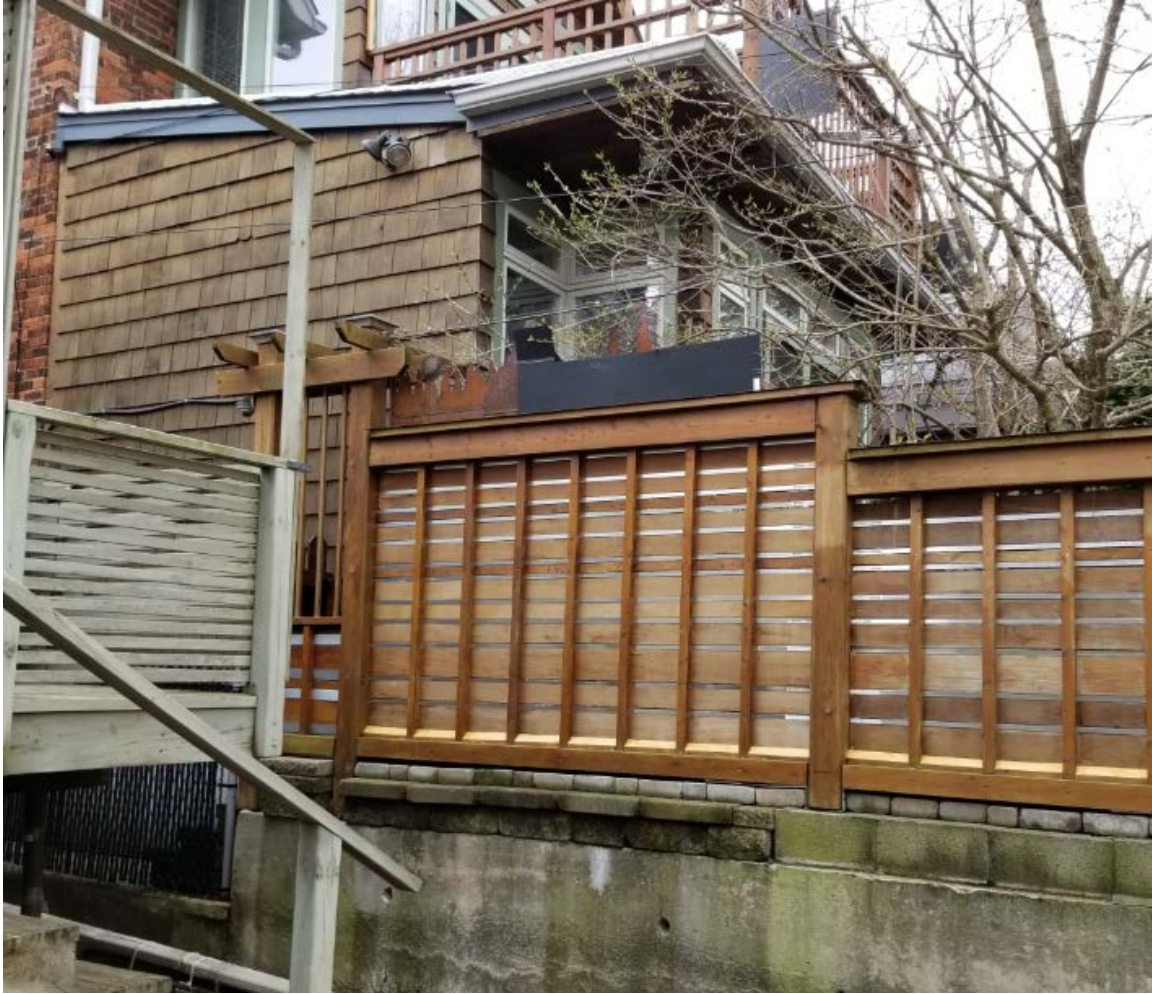
Retaining wall measures 1.04 metres with a 1.6 metre wooden fence panel attached on top.
