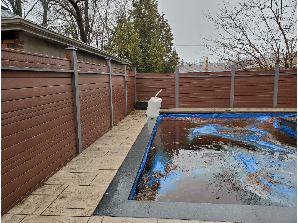
Attachment 5: Rear Yard Fence of 8 Darien Court, North / North Western exposure
