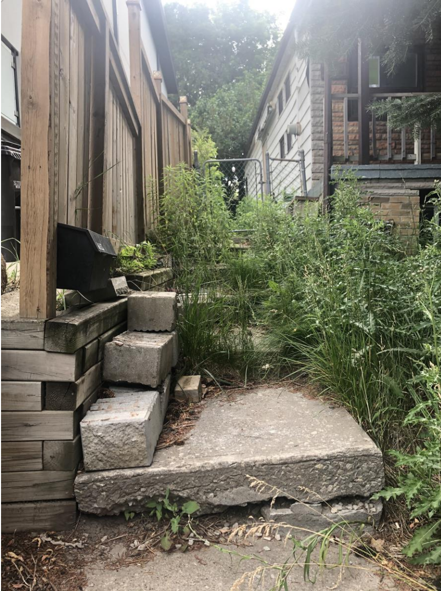
This picture depicts the current condition of the concrete steps that are within the city's road allowance.
