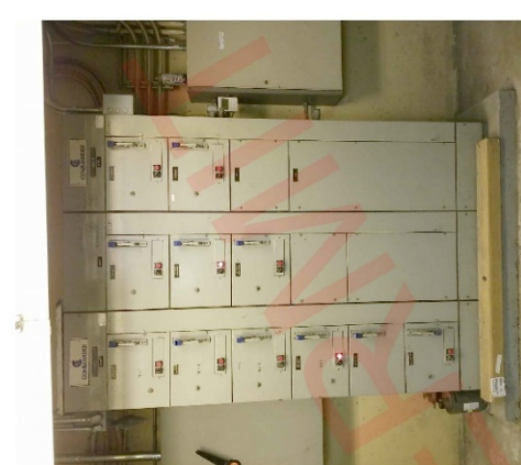
2 CP58.3 ELECTRICAL SWITCH BOARD
